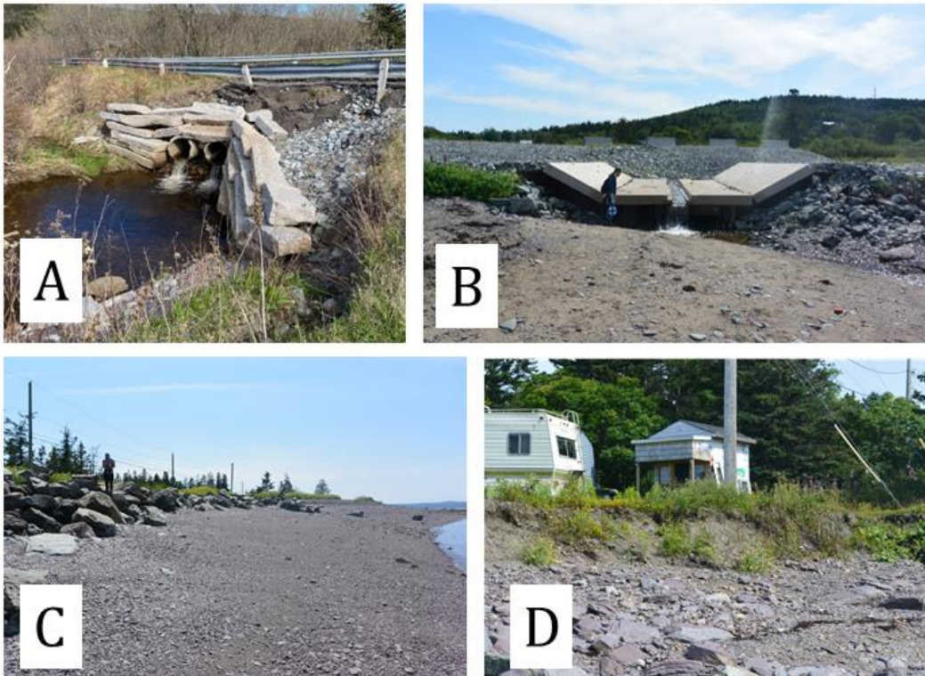
Figure 12: Example of form types at Anthony's Cove. (A) Anthony's Cove culvert in AC10 showing cracking of Anthony's Cove Road. (B) Bean Brook culvert in AC7. (C) Riprap protecting roadway ends in AC14 and begins again in AC17. (D) Erosion near utility pole at AC23.
