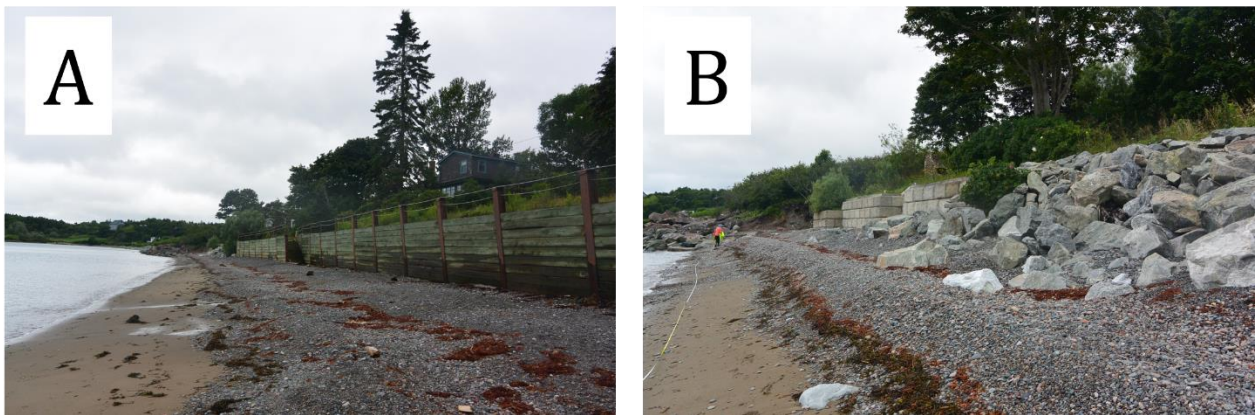
Figure 34: Images (A) Wooden seawall in MCB4. Staircase shows signs of wave damage and wall is angled towards the shoreline indicating erosion is occurring beyond the protection. (B) Concrete seawall and riprap in MCB5 to protect homes.
