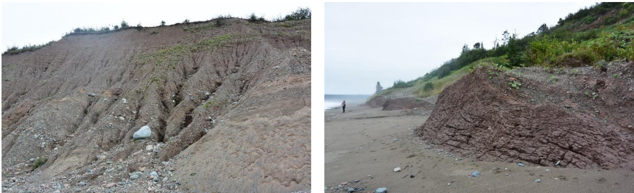
Figure 40: Images: left, drainage channels and loose boulder material in SP10. Soil layers visible at the top of the slope. Right, multiple slumps in the backshore at SP11.
