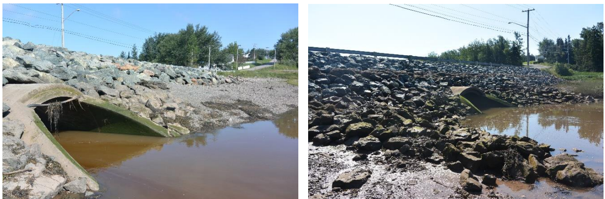
Figure 48: Images: left, culvert at LVPO1 on the coastal side of the roadway. Bottom, at LVPO2 on the inland side. Culvert appears to be in good condition.
