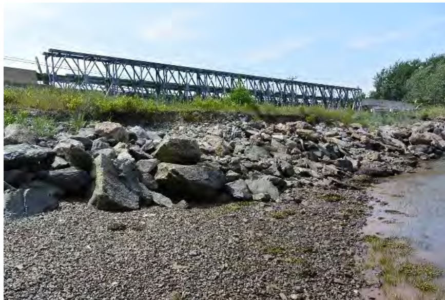
Figure 13: Riprap protection has been installed around Lorneville Cove to reduce erosion during periods of high water. Monitoring erosion along this infrastructure will be required to ensure it continues working as storm events intensify throughout the century.
