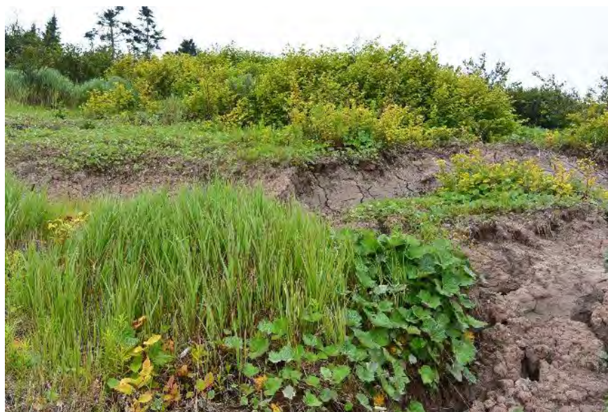
Figure 14: Mass movement occurring along the Sheldon Point Trail which is displaying multiple mass movement events as there are two exposed bluff faces identified in this image (ACAP Saint John, 2016).
