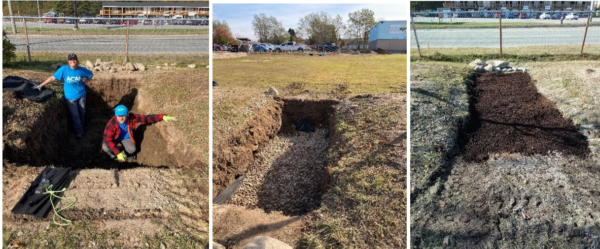
Figure 5: Infiltration trenches installed at Glen Falls School. Left: Full depth of 3ft was removed. Middle: Rock was filled at the base, to increase infiltration. Right: Sand was filled in with topsoil and grass seed.
